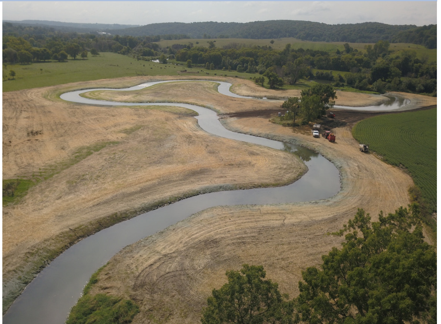
MILL CREEK POST-PROJECT. NOTE THE NEWLY NARROWED CHANNEL, SLOPED BANKS, AND FLOODPLAIN ACCESS. SOILS ARE STABILIZED WITH HYDROMULCH AS COVER CROP BECOMES ESTABLISHED. (PHOTO: PAUL KRAHN TU DARE)
