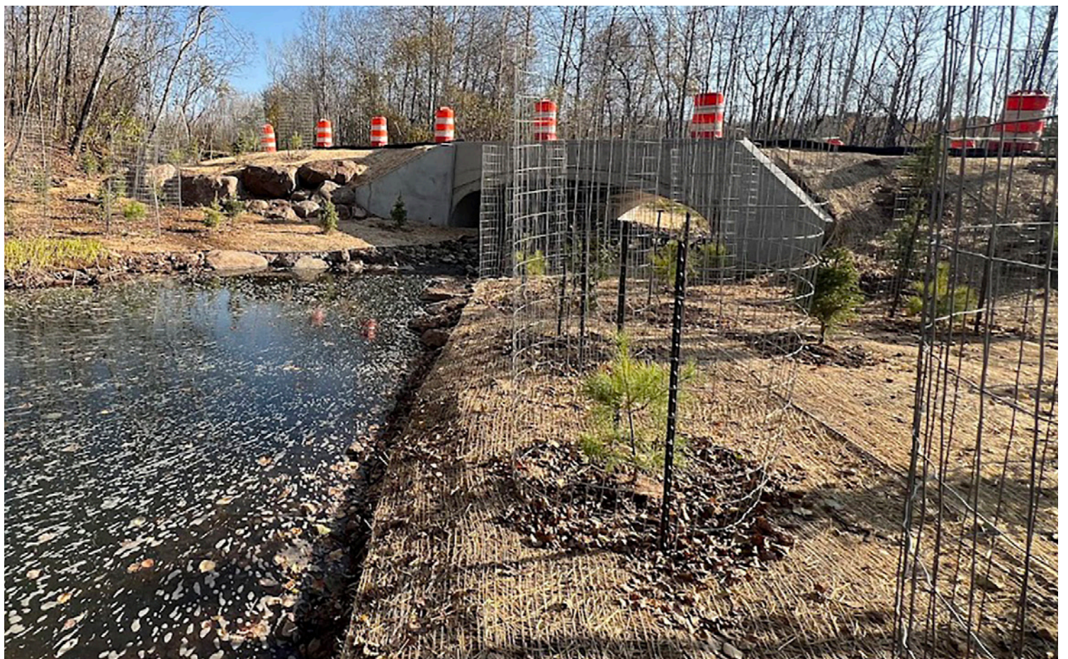
KEENE CREEK (OKERSTROM ROAD, HERMANTOWN). A LARGE POOL BELOW THE NEW CULVERT CONTAINS TOEWOOD AND BOULDER HABITAT, AND NEW NATIVE TREES PLANTED IN PROJECT AREA WILL PROVIDE WILDLIFE HABITAT AND FUTURE SHADE.
