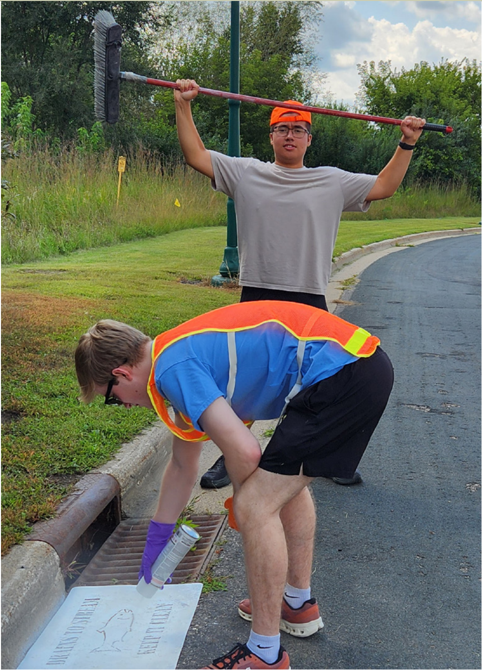
SKYLER SPRAY-PAINTED STENCIL MESSAGES AS A REMINDER THAT STORM DRAINS FLOW INTO STREAMS.
